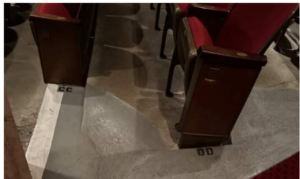
Access to & from aisles creates a hazardous condition
